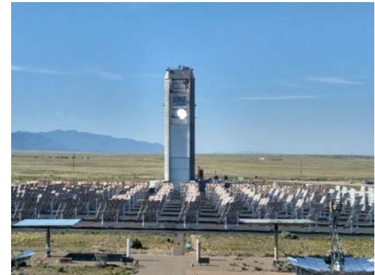
Fig. 1. On-sun testing of the bladed receiver design at the National Solar Thermal Test Facility, Sandia National Laboratories, USA.
